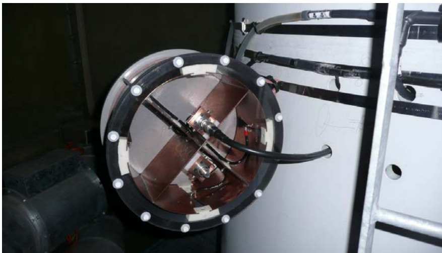
Figure 3.16. Installed B-dot sensor and Rogowski coil around the inner metallic structure of the tower, upper measurement location (82 m).
