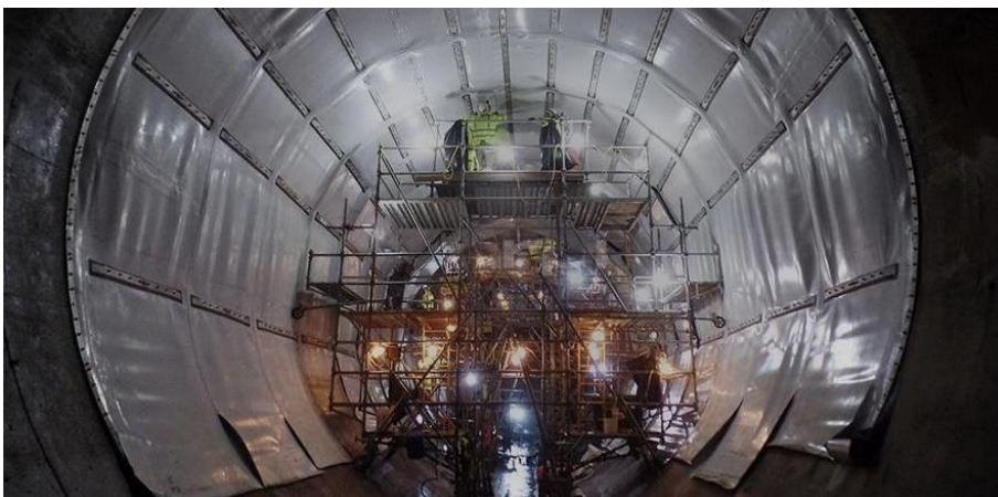
Figure 12: Installation of a geomembrane system in a pressure tunnel. Image: courtesy of © Carpi Tech
