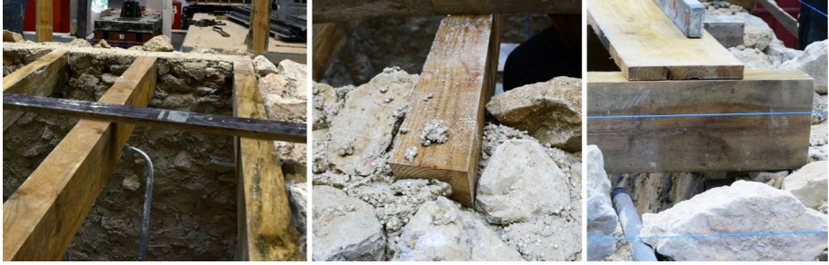
Fig. 7 Beam supports at the 1 st floor of Unit 2 of the masonry aggregate specimen
