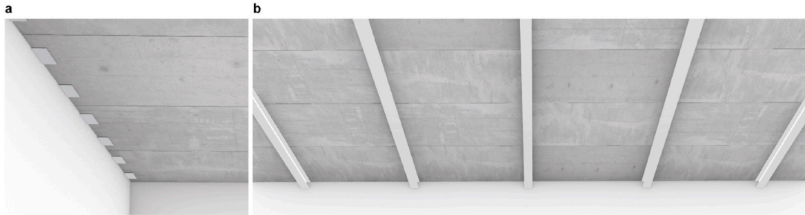
Fig. 5. Low-angle views of the two systems: (a) System A and (b) System B.
